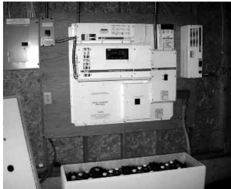
Power panel with battery box
