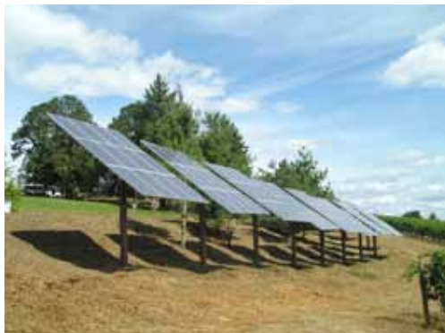
Fixed ground mount at Sokol Blosser Winery
